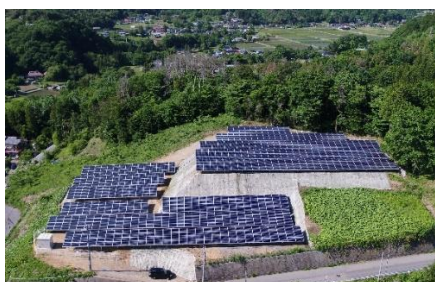
Gunma Prefecture Power Plant
